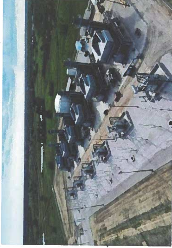
Sample 300 MW fast acting natural gas facility
